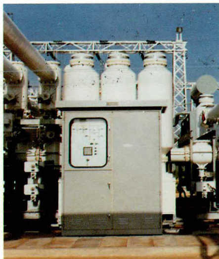
Peralatan 275 kV dalam pencawang Skudai. 275 kV equipment in Skudai substation.
